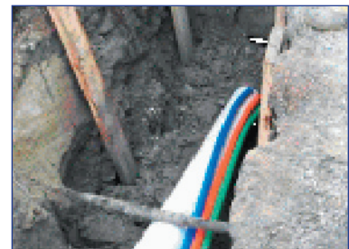
Fig 3: Beginning deployment of the rugged new HDPE pipe (white) and fiber-optic conduits (multi-colored). Photo courtesy of RIS.
