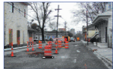
Fig 2: With pipe-bursting technologies, little excavation is required for deployment; here, only a few cuts have been made in the pavement for deploying lateral connections from the main line directly to buildings. (Photo courtesy of RIS: New Orleans CBD deployment.)
