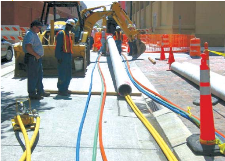
The City of New Orleans is upgrading its telecommunications system in its central business district by using dual-purpose rehabilitation to install fiber-optic ducts while simultaneously replacing its aging sewer mains.
